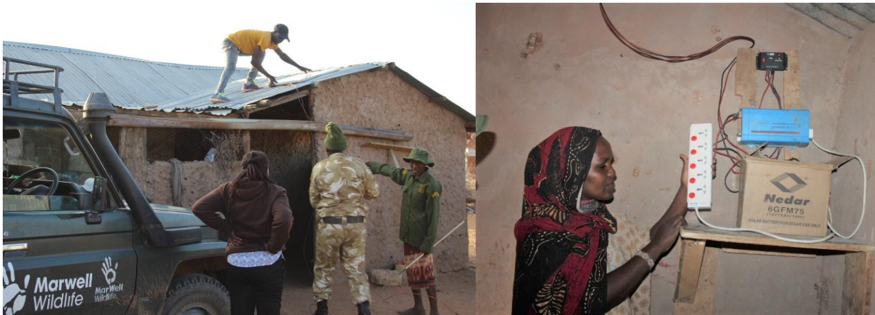
Pictures 40 & 41: Installation of solar panel in Kargi (left) & training Mogor in charging system maintenance © Marwell
